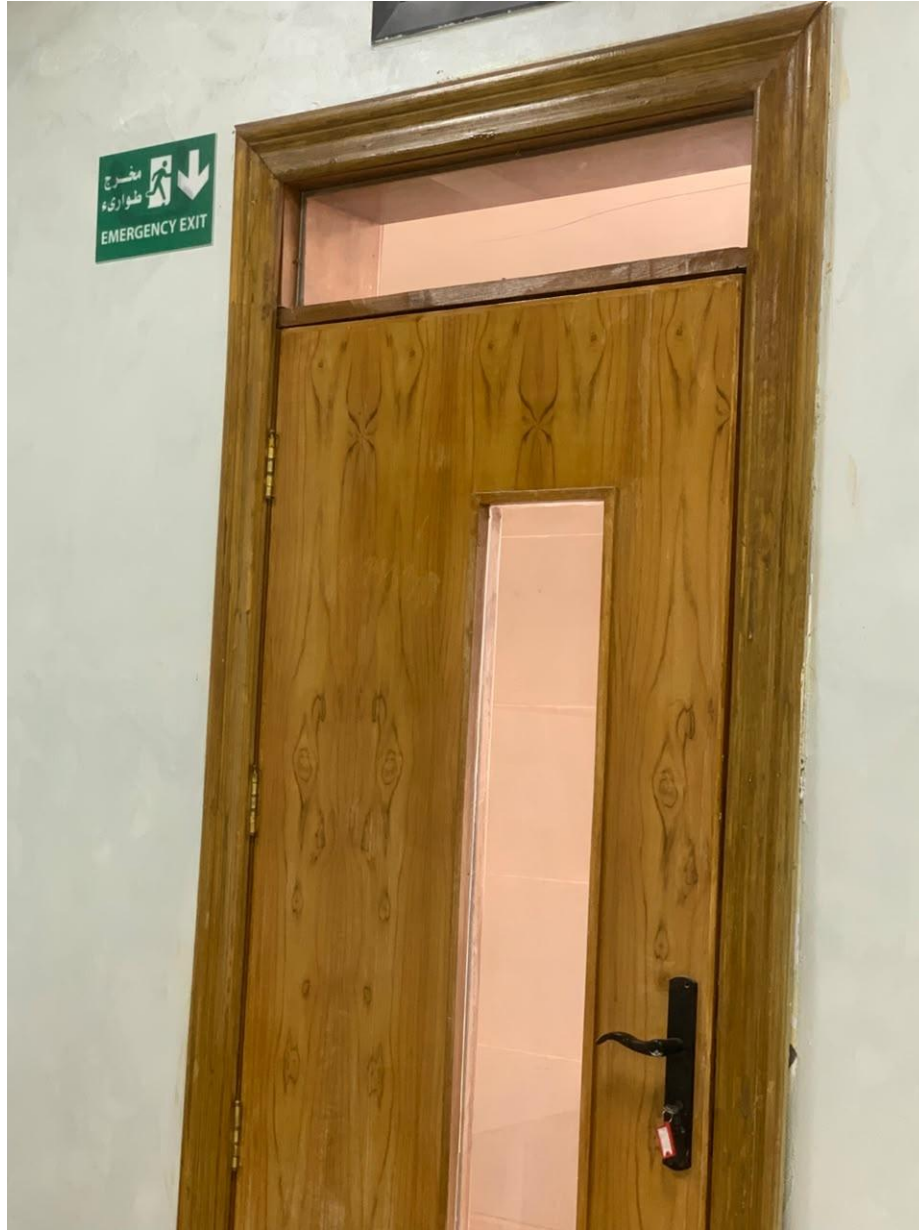
Figure 2.1.6g: Dedicated Emergency Exit wooden door equipped with panic hardware and an illuminated green safety sign ('EMERGENCY EXIT / مخرج طوارئ').
